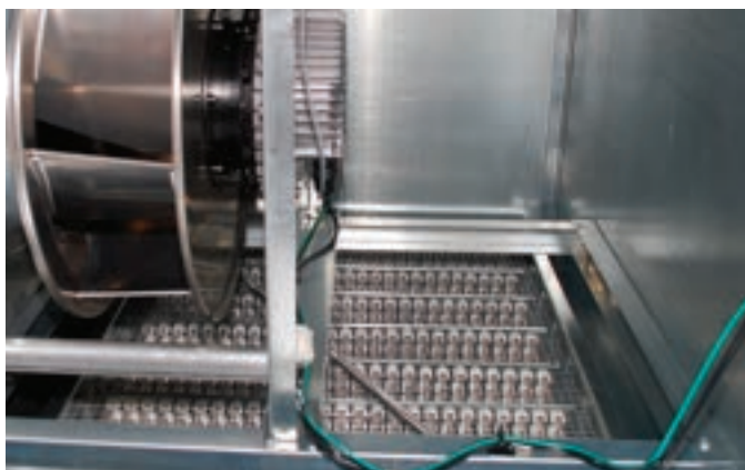
Figure 8: Electric Heat Coils
