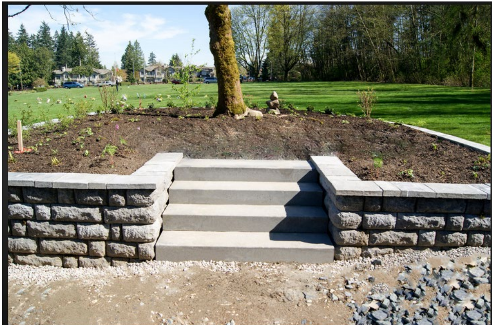
Here is an example of the concrete step. we only need one since the patio is so low to the ground. It will be a standard size and shape-36" wide.
