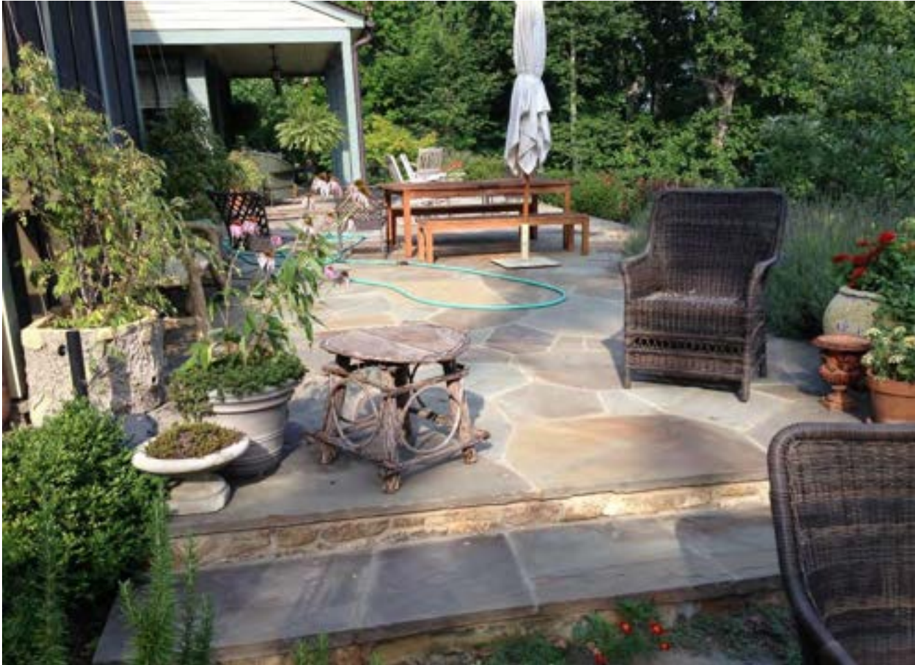
Flagstone Patio – Irregular shaped Pattern, not too much cleft, 2” thick edge pieces and step treads, Fieldstone Step Risers. Patio to be set on 4” thick reinforced concrete slab with mortar joints.
