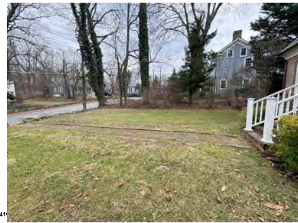
Existing Front Brick Lead Walk to be Reset because it sunk
