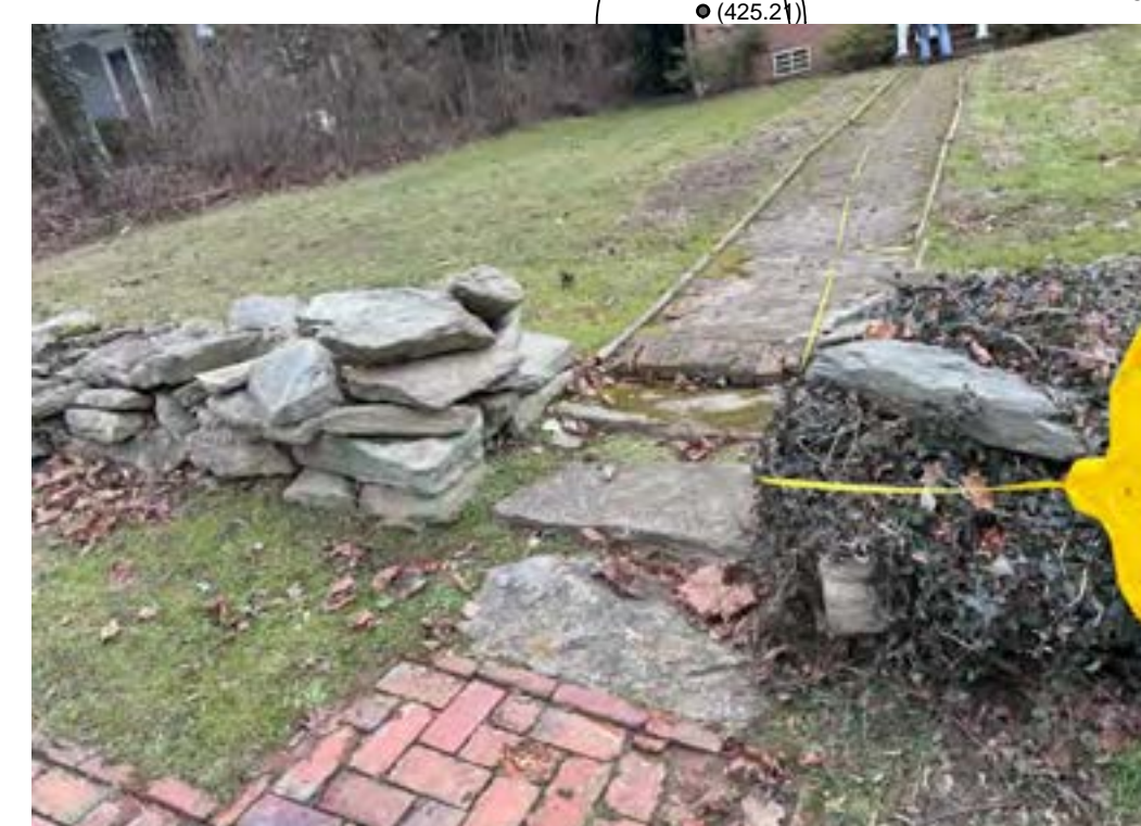
Existing Stone Wall to be Re-stacked and Reset Top Brick Step and/or Stone Step = TBD onsite w/ Mason
