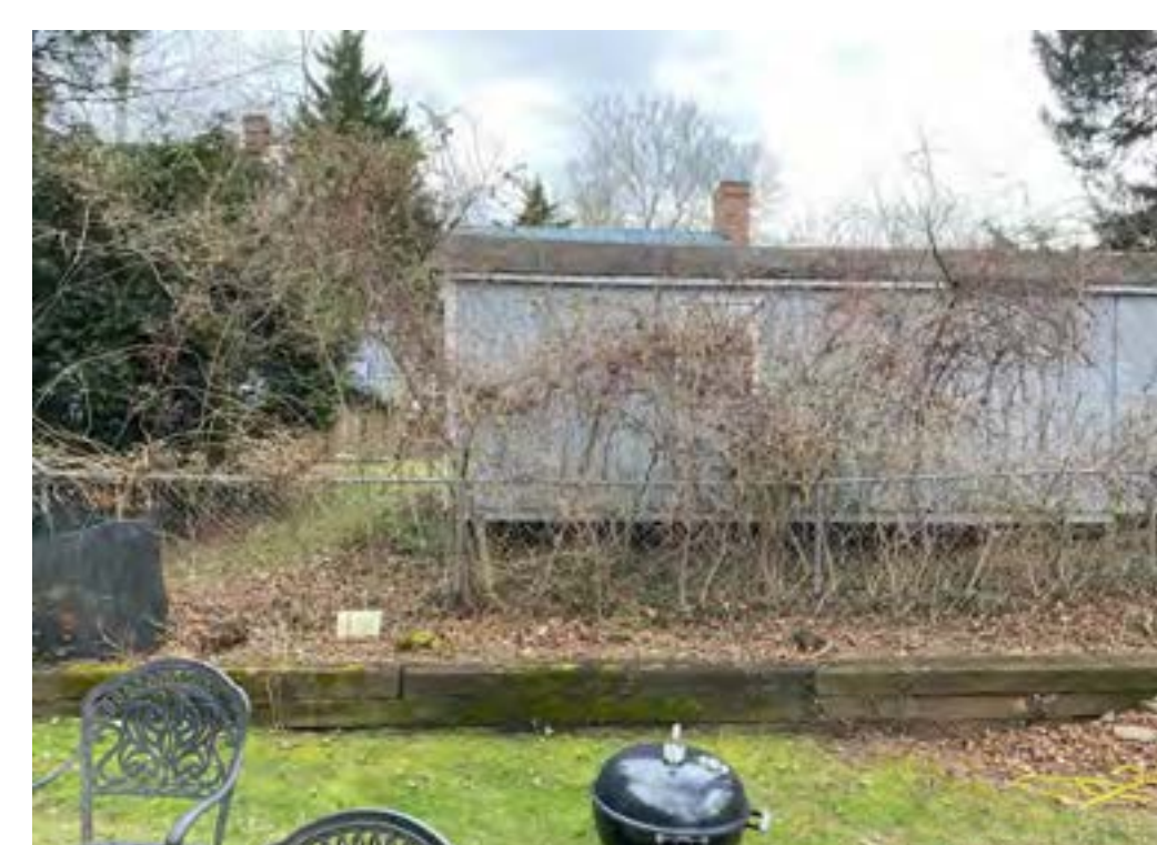
Partial view of Existing Timber Retaining Wall to be Replaced w/ 6x6 P.T. Timbers
