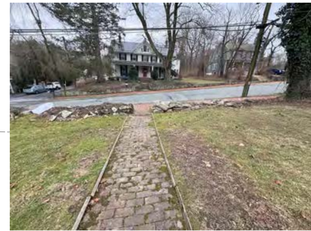
View of Brick Front Walk and Existing Stone Wall. Wood Edging along Brick to be Removed. Brick walk to be Slightly Raised + Reset.
