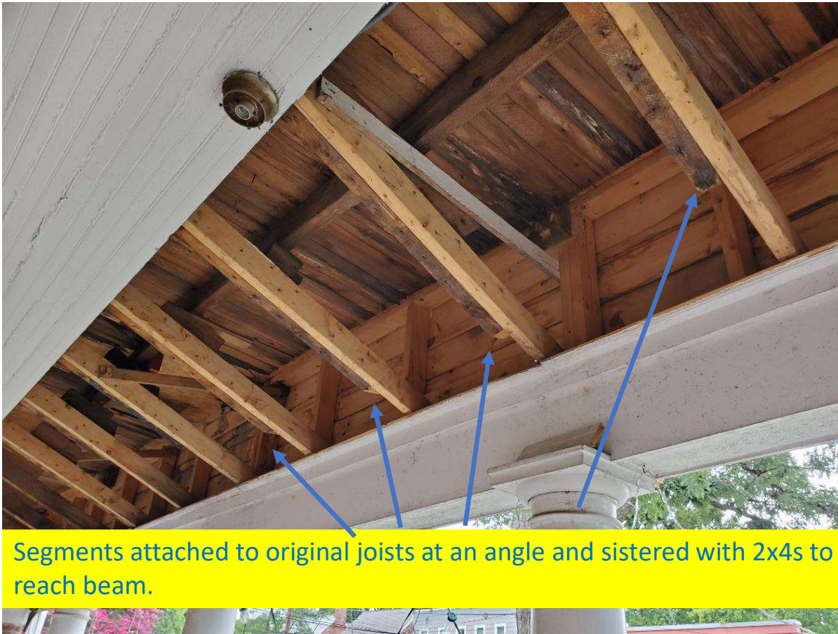
Photo 1 - 7102 Maple Ave – cut joists too short
