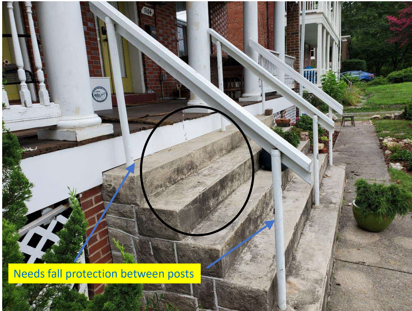
Photo 14 - 7102 Maple Ave – steps showing no fall protection
