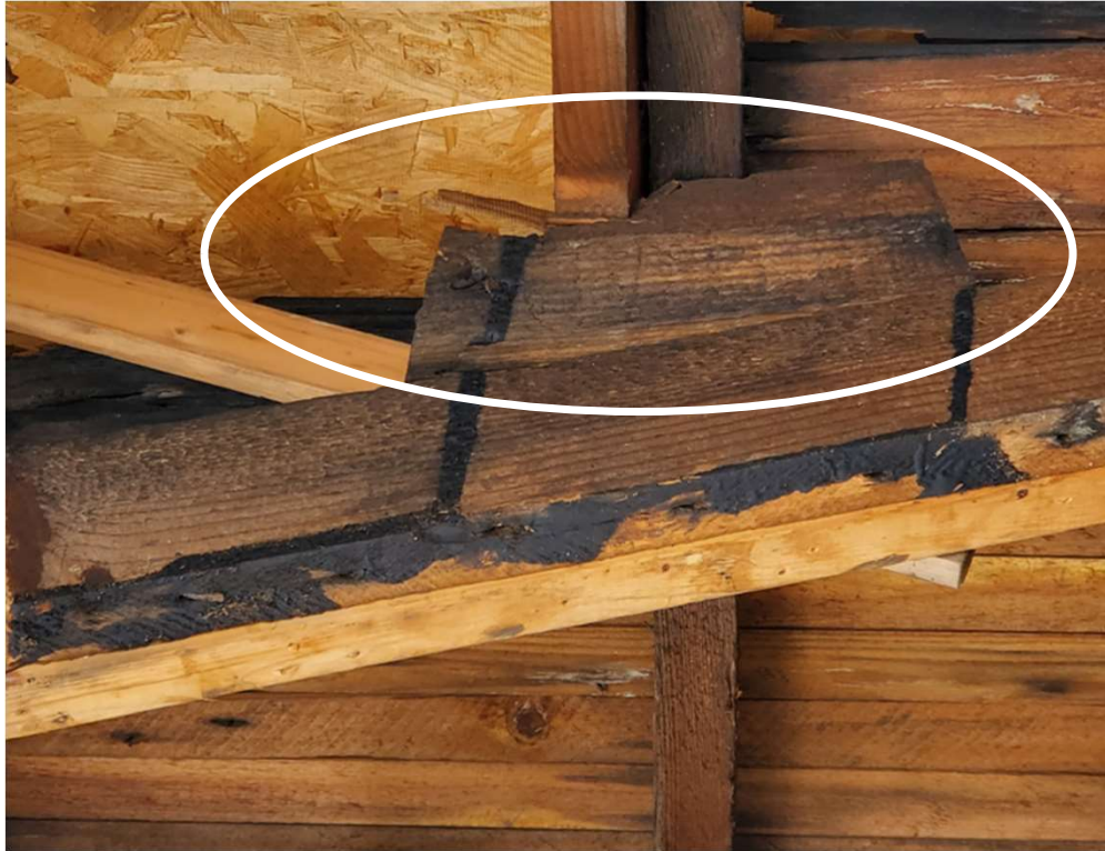
Photo 5 - 7102 Maple Ave – odd shaped shims holding up 20 Foot long 2x4s
