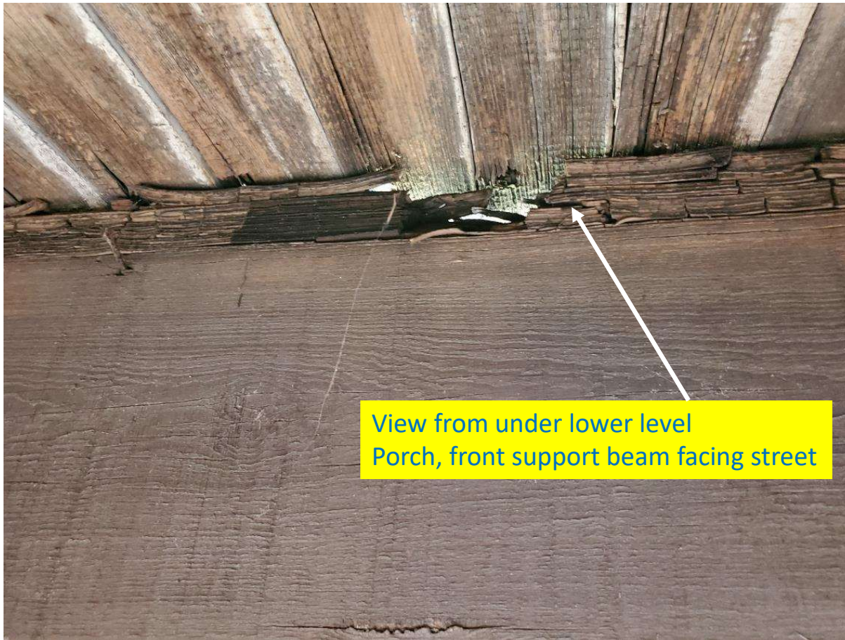
Photo 11 - 7102 Maple Ave – lower porch floor joist rot
