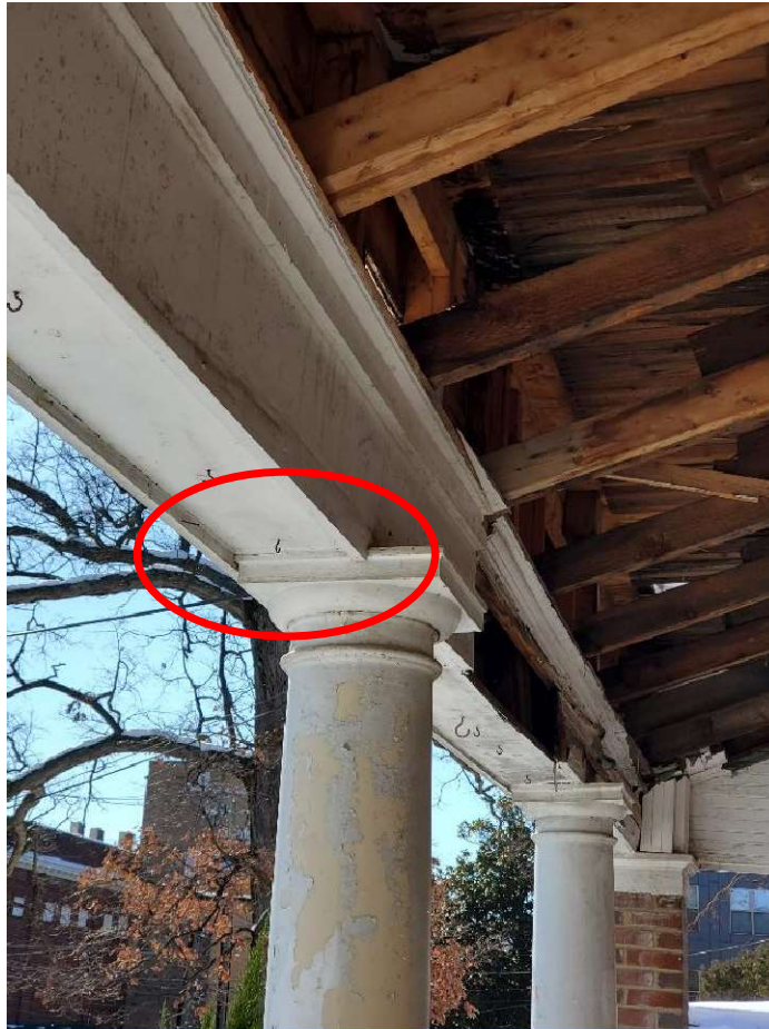
Photo 10 - 7102 Maple Ave – off center beam
