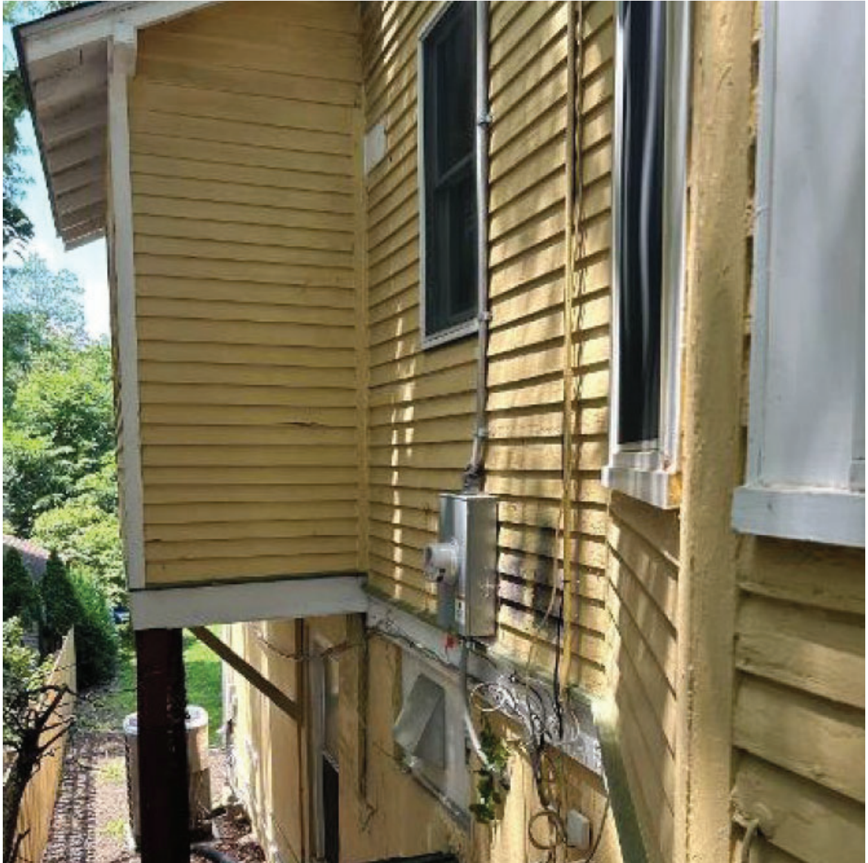
Utility Meter before Installation
