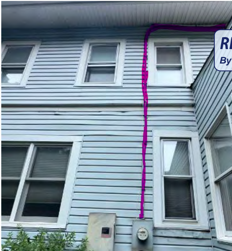
Utility Meter after Install
