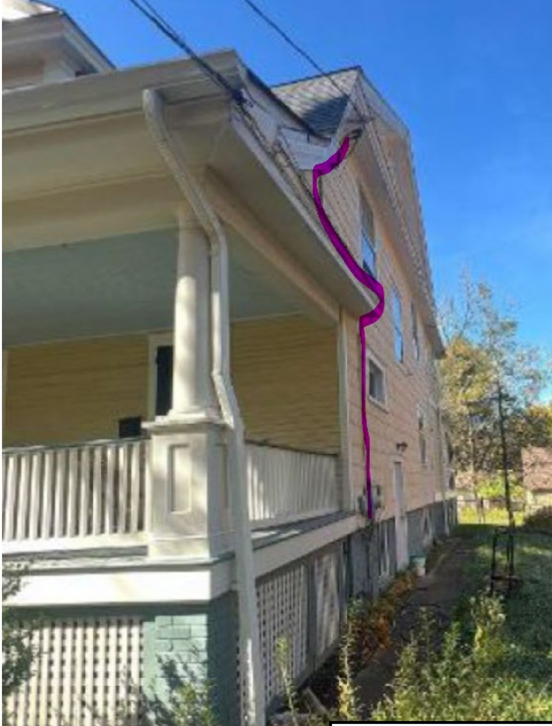
Utility Meter after Install
