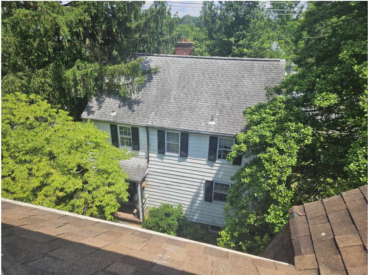
Western face of roof as viewed from 2nd floor window of 3906 Washington Street
