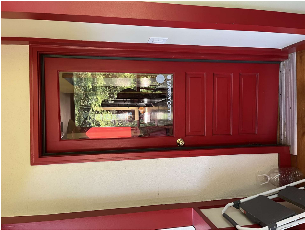
EXTERIOR DOOR LOCATED IN THE KITCHEN AT THE REAR OF THE PROPERTY, ENCLOSED BY PORCH, TO BE REPLACED.
