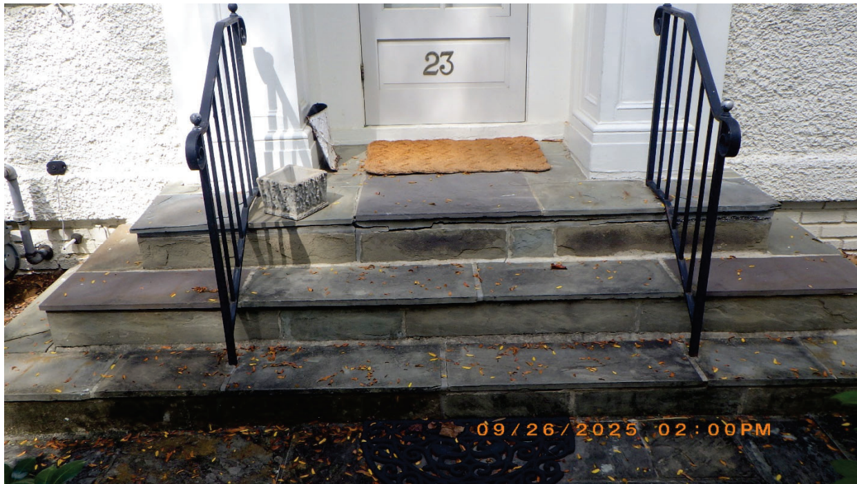
Figure 2. Existing front portico/step to be replaced
