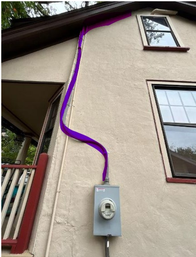
Utility Meter after Install
