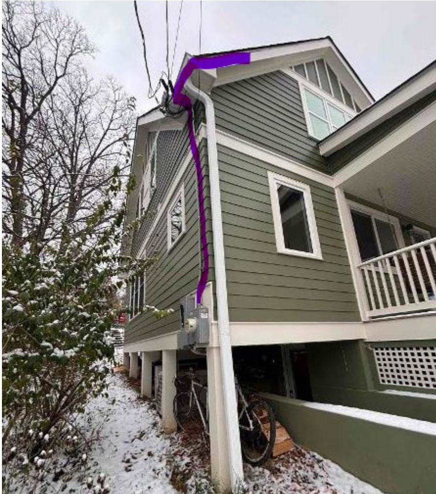
Utility Meter after Install
