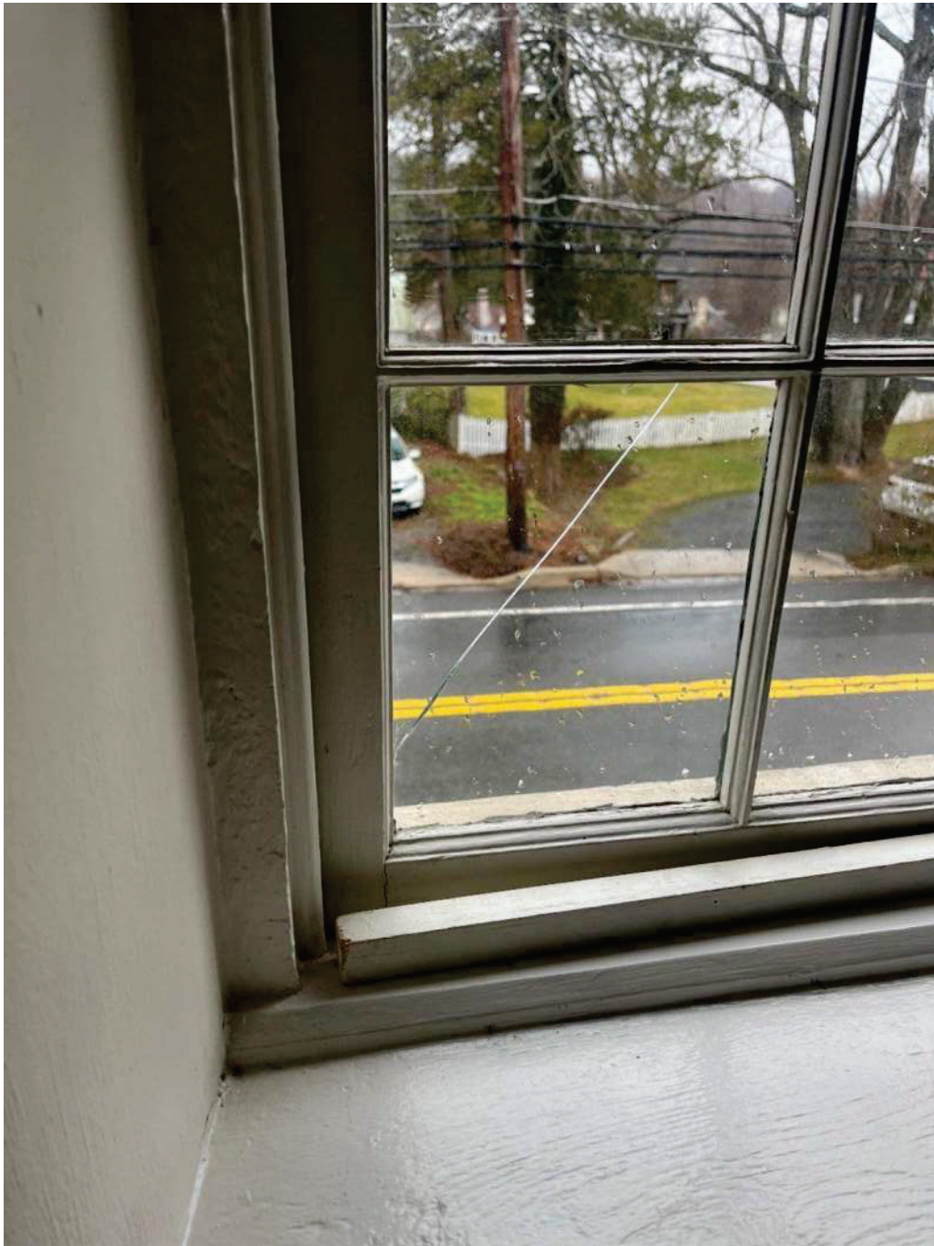
Photo 48 - Window Close-Up Showing Broken Glass
