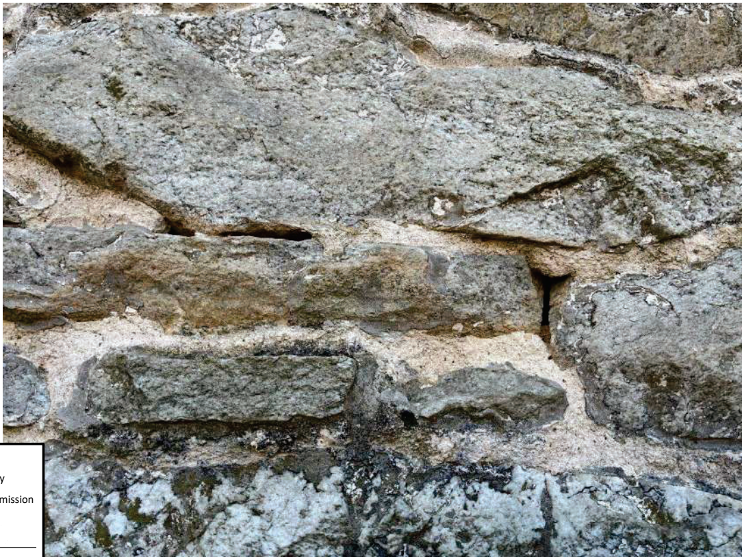
Photo 23 - Masonry Façade Close-Up Showing Missing Mortar
