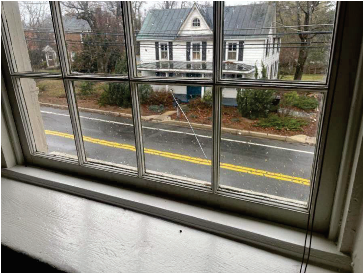
Photo 47 - Window Close-Up Showing Broken Glass
