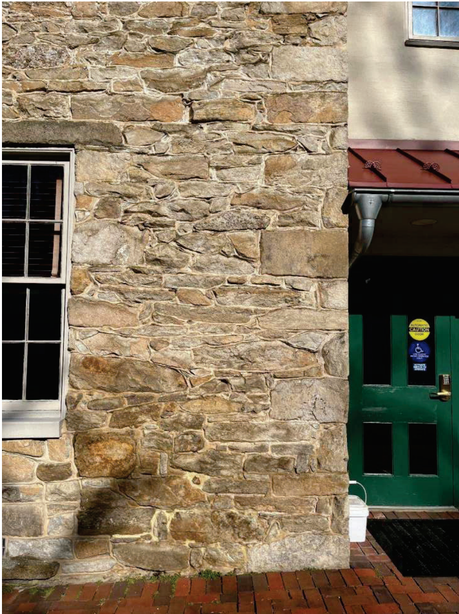
Photo 18 - Masonry Façade Showing Moisture
