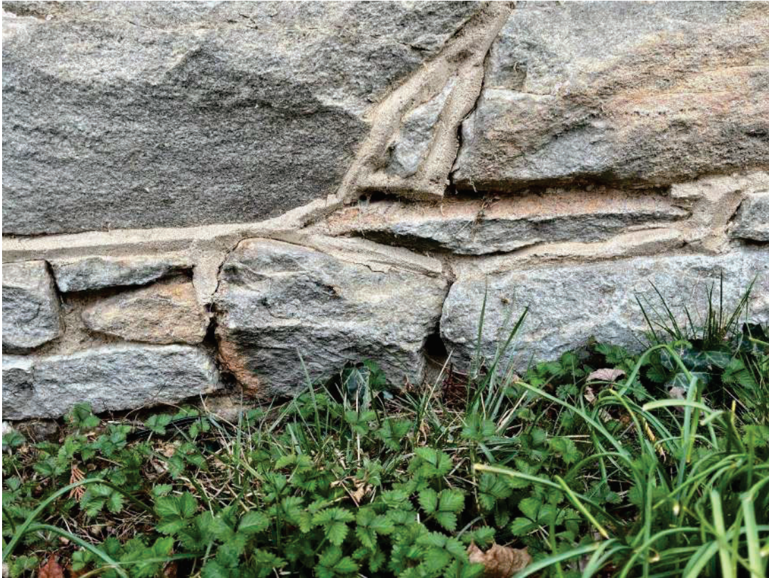
Photo 24 - Masonry Façade Close-Up Showing Missing Mortar
