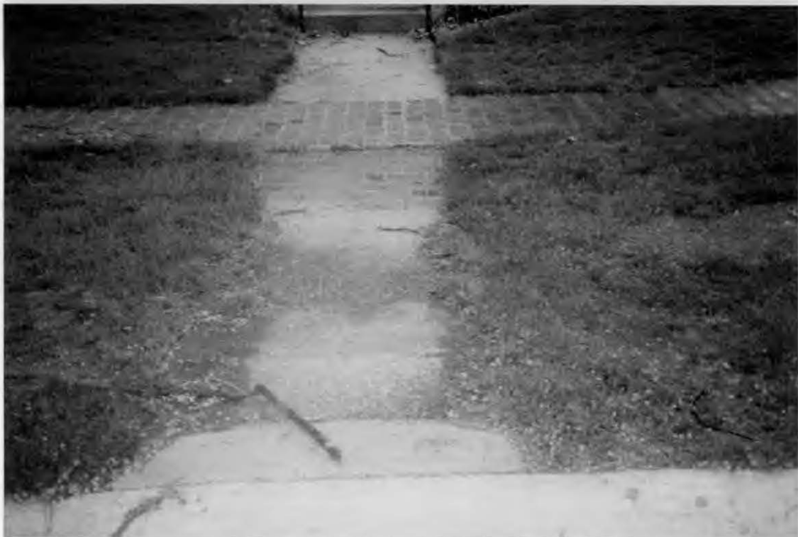
Close up of walk from street curb to city sidewalk - #7 East Melrose
