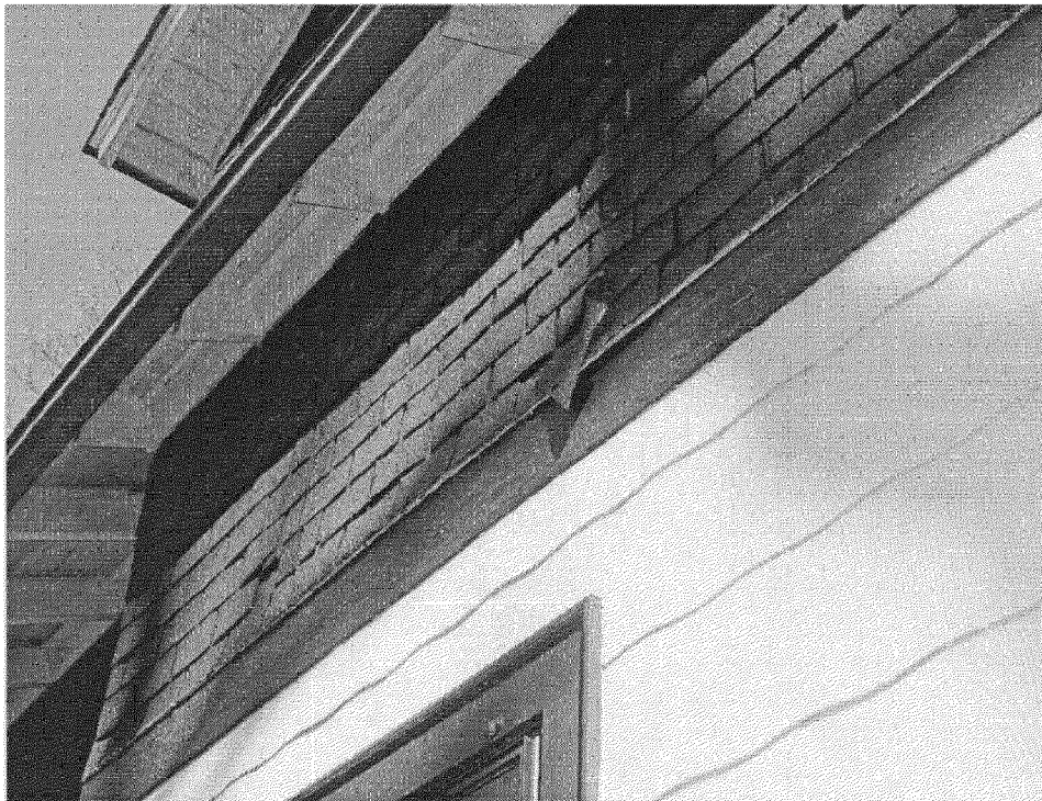
Asphalt shingling on upper wall showing damaged shingle, with asbestos siding below
