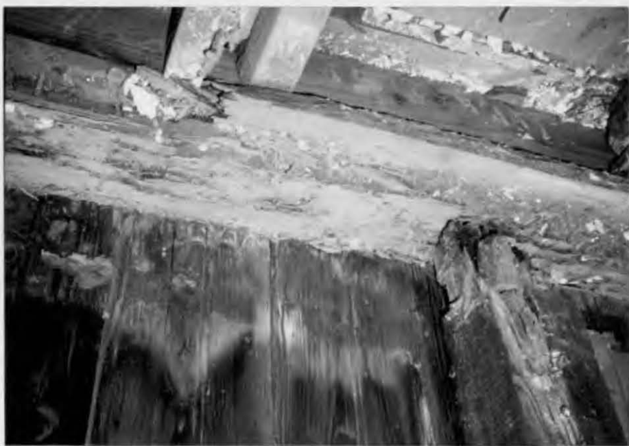
TERPITE; WATER DAMAGE TO SUPPCH 7119 WILLOW AVENUE TAYLOR PARK, MD
