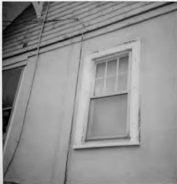
Patch - 7112 Sycamore Ave, TP window will not hold paint - ventilators installed.
