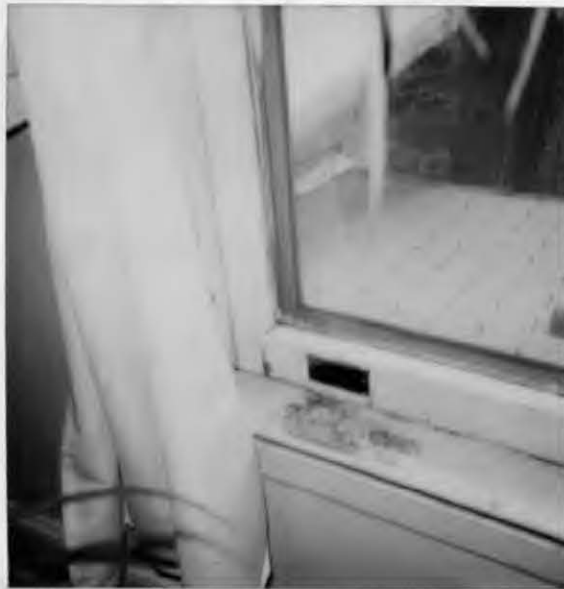
Patch, 7112 Sycamore Ave, TP wood damage, rot rust damage from window trim
