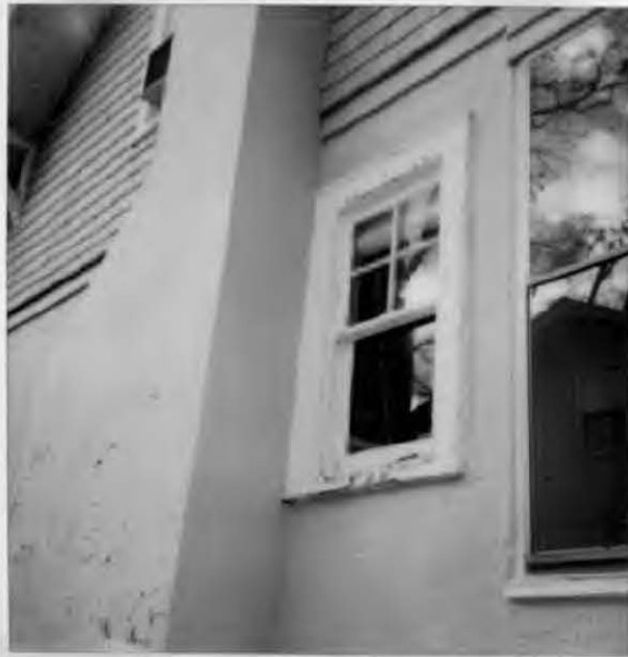
Patch, 7112 Sycamore Ave, TP window will not hold paint or putty
