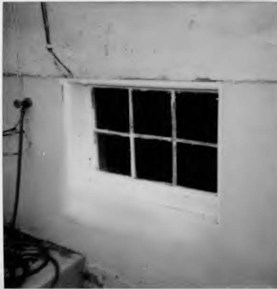
Patch, 7112 Sycamore Ave, TP window will not hold paint/petty. basement level
