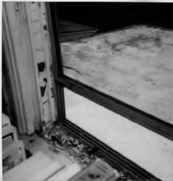
Patch, 7112 Sycamore Ave, TP window will not hold paint rot
