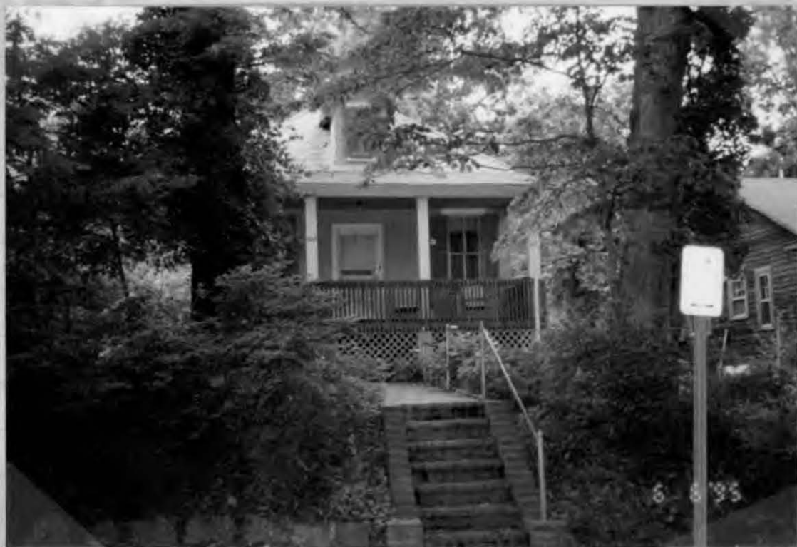
Shows ③ Wood Pillars ④ Front Stairs to Left ⑤ Wood Railings
