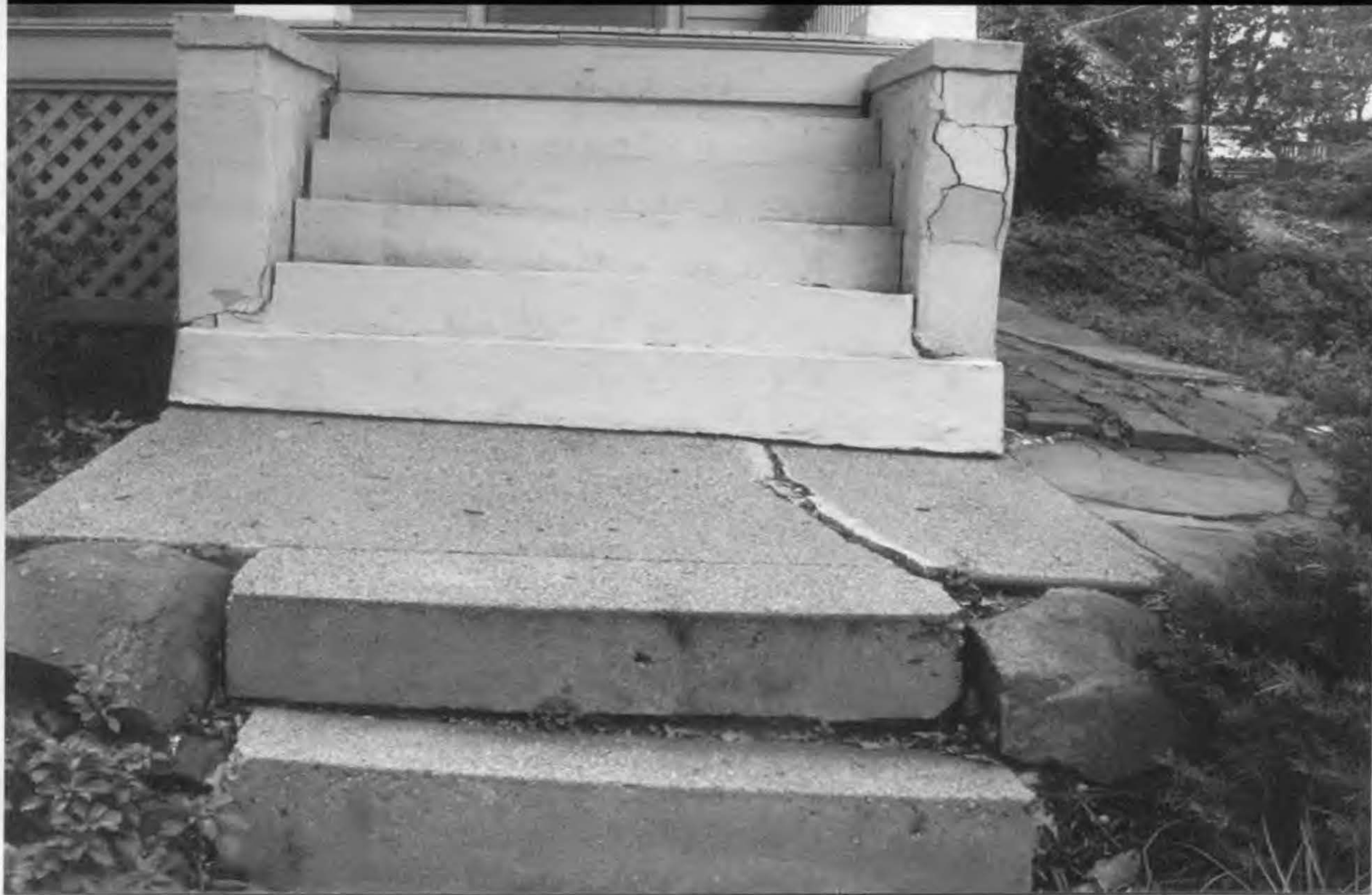
Photo 7: Structural Damage to walkway steps, apron, and porch steps due to settlement on steep slope at front of house.
