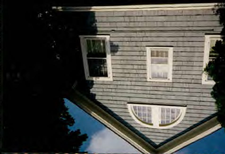
DETAIL: WEST FACADE - AFFECTED WINDOWS
