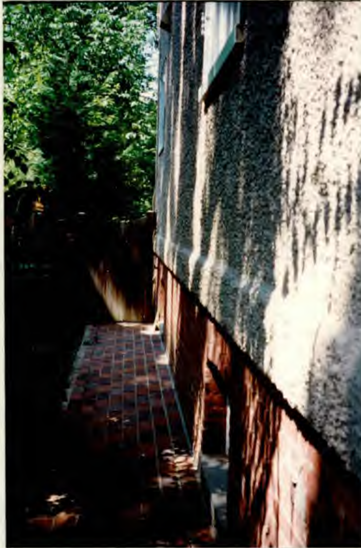
LEFT SIDE OF HOUSE WITH EXISTING GATE (Remove gate and install new one)
