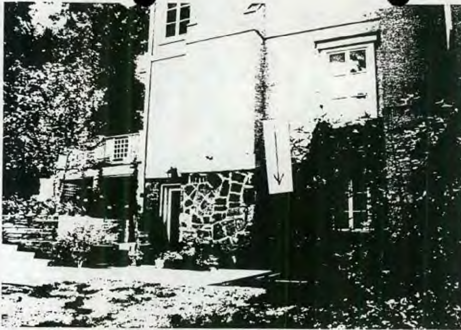
Photo #7 - West wall showing location of new window; Location of PART "D"
