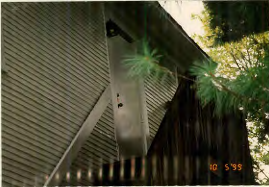
REAR VIEW- UPPER DOOR TO BE REPLACED WITH WINDOW TO MATCH EXISTING WINDOW TO LEFT (see below)
