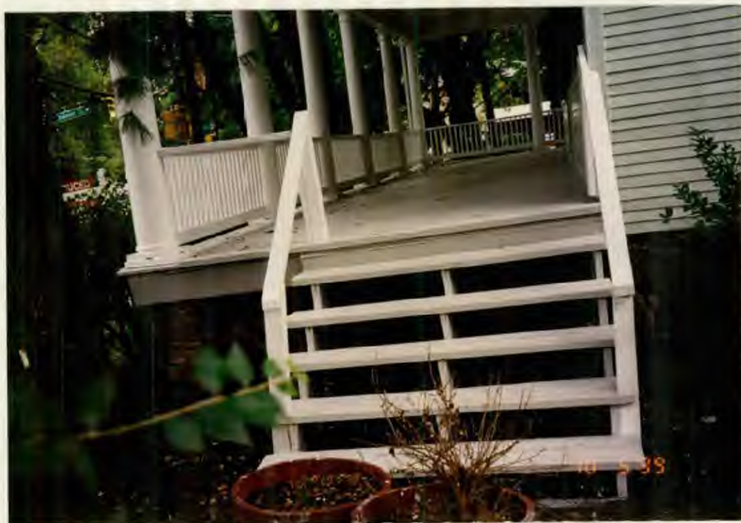
FRONT PORCH VIEW- STEPS TO BE REPLACED WITH PAINTED TREADS & RISERS (TO MATCH PORCH) WITH PORCH RAIL TO MATCH EXISTING
