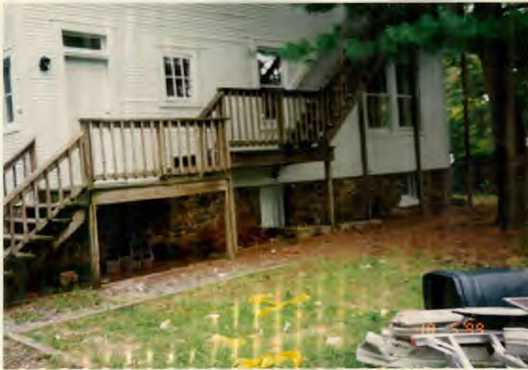
REAR VIEW- AREA FOR NEW DECK (See Attached Plan) STONE FOUNDATION TO REMAIN EXPOSED WITH NEW DECK
