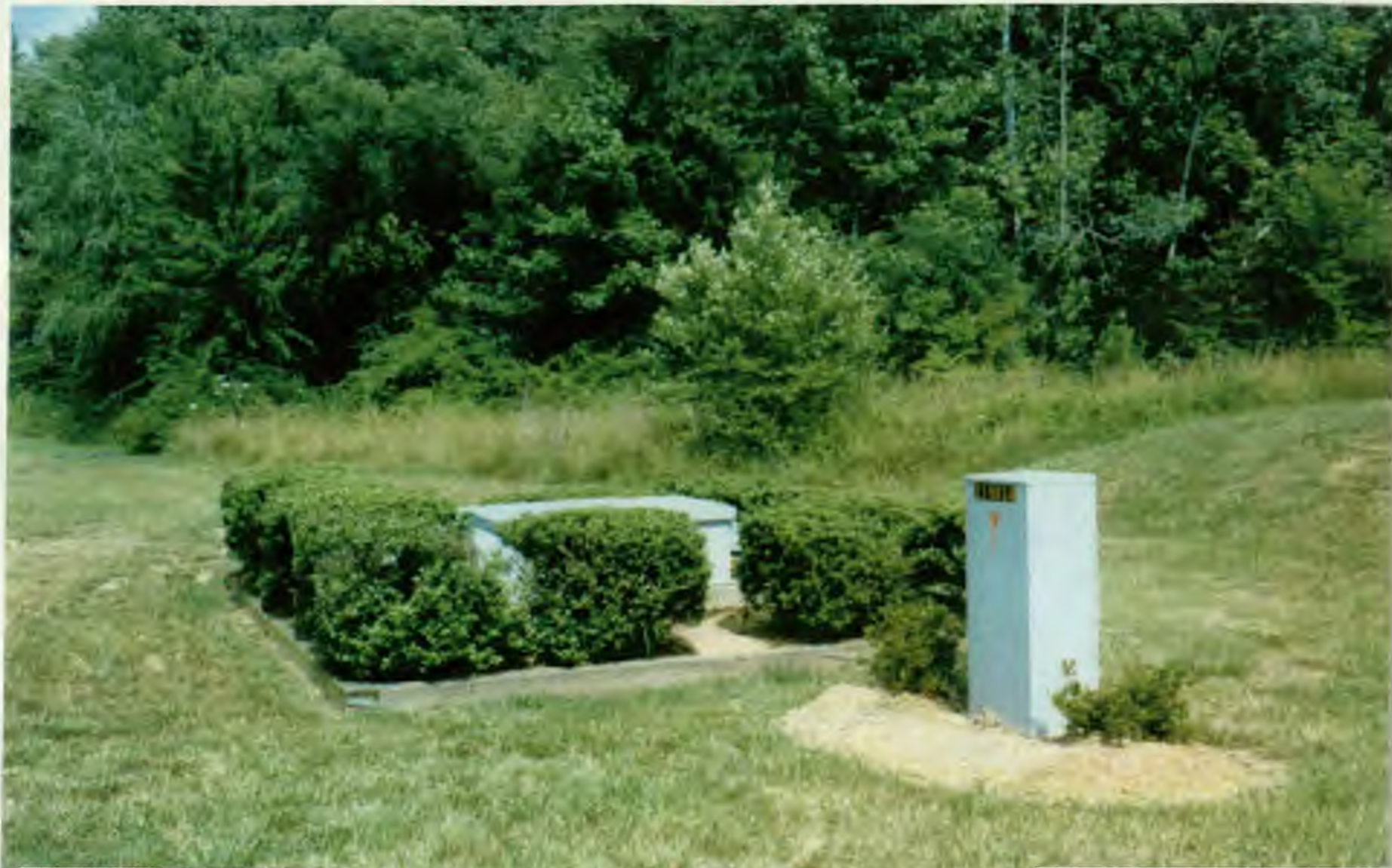
Typical CEV (Controlled Environmental Vault) - Shown with electric meter pedestal
