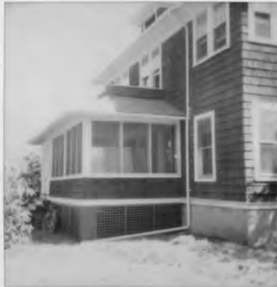
FRONT PORCH JALOUSIES TO BE REMOVED
