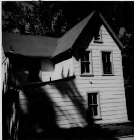
Bank of house in '94 before addition of french door + windows as Approved by HAWP.
