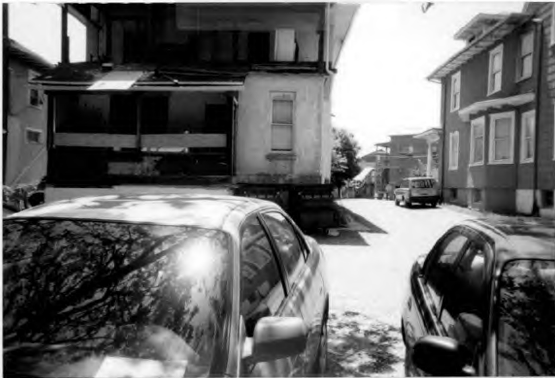
Rear of 7034 Carroll Ave Showing existing, deteriorated wooden porches to be replaced with new addition.
