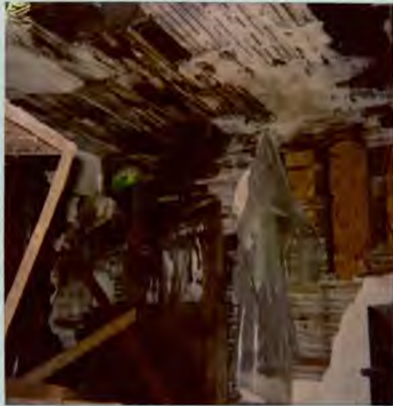
6-19-90 4722 Dorset 1 fl rear water + fire damage
