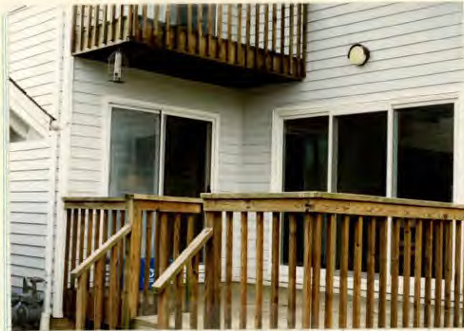
Double sliding door is to be replaced
