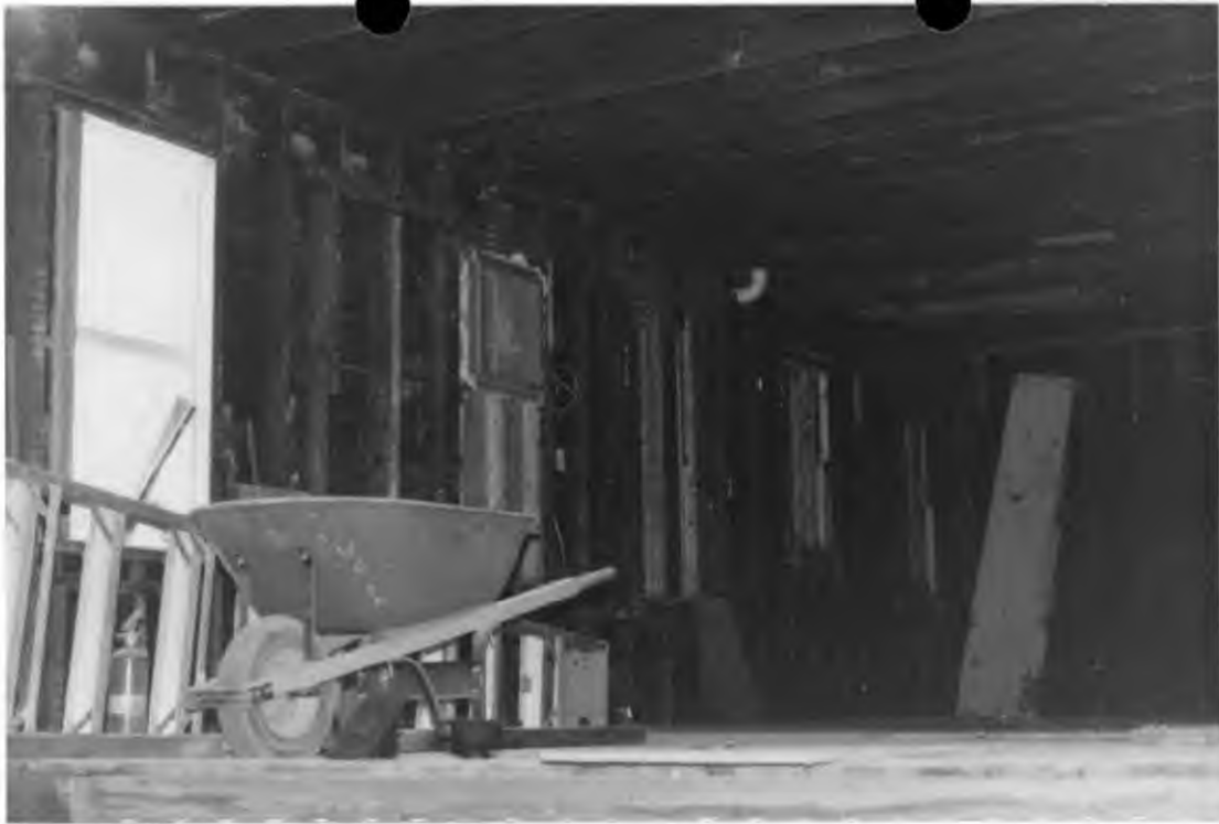
View of top floor left/rear from front of building. Would like to restore one or two windows on this side.
