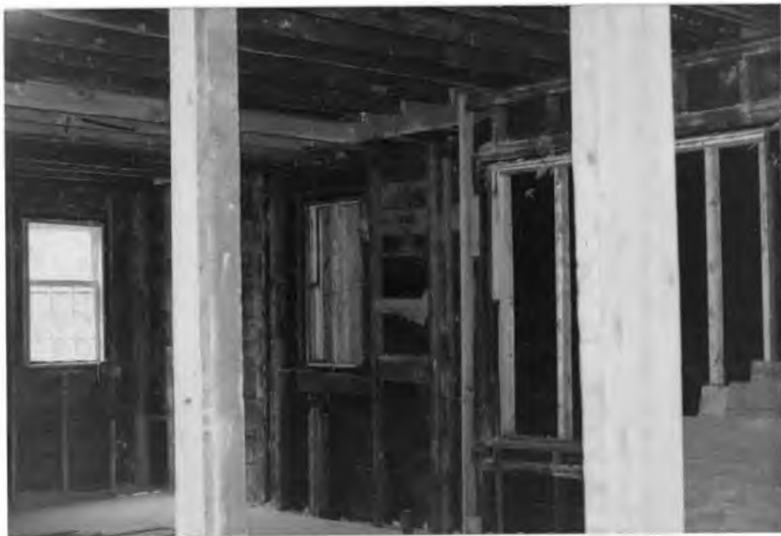
View of top floor right/rear from front of building. Open window at left in the photo faces rear of property. Would like to restore one or two windows on the right side of building.
