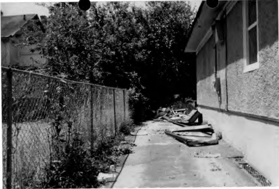
View of left side of building adjoining 1 Columbia Ave. Fence to be replaced by 6' wood. One or two windows to be restored.
