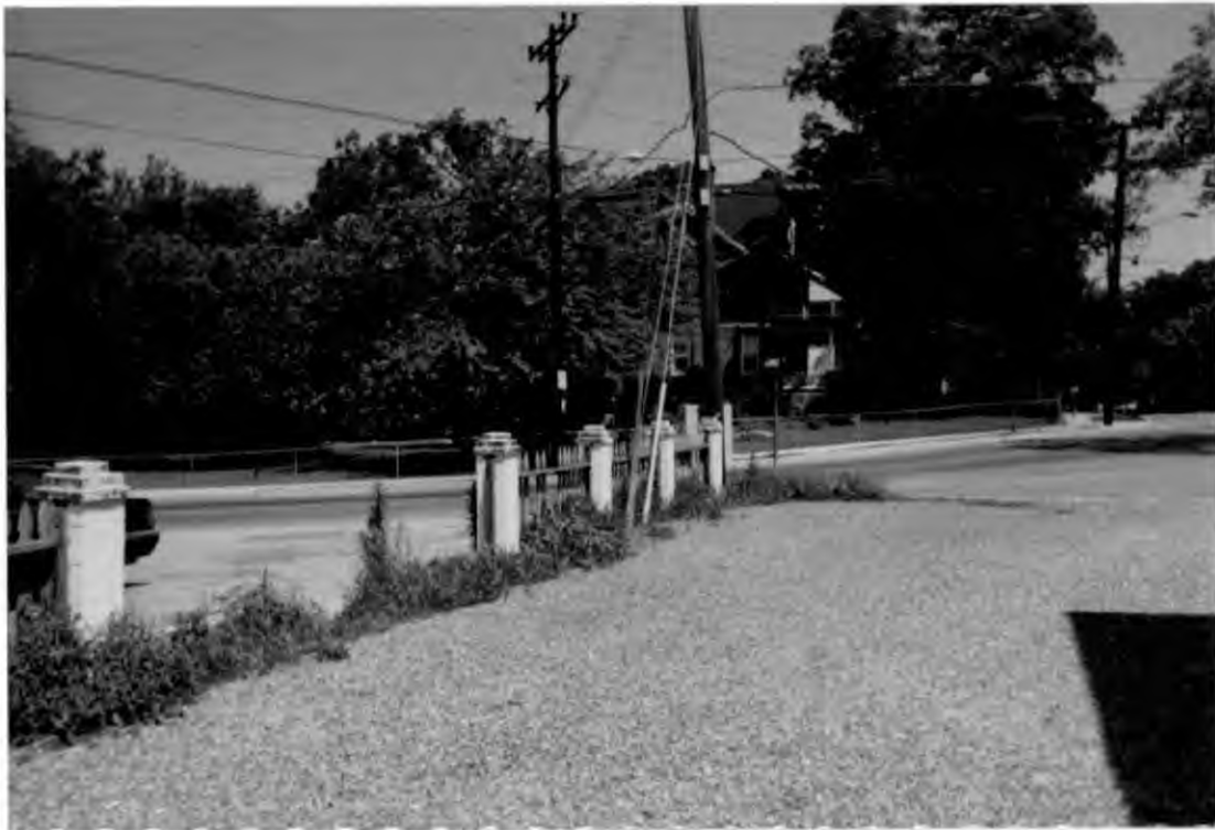
Fence to be repaired/restored between property and parking area of 1 Columbia Ave. Six-foot wood fence will begin/connect at face of building. House shown across Carroll Ave. is 102 Park Ave.
