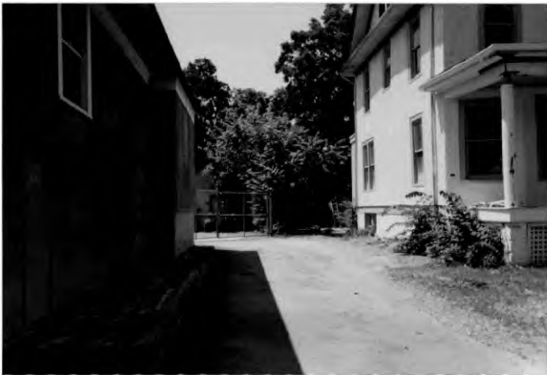
View of right side of building from front. One or two windows to be restored. Chain link gate to be removed.
