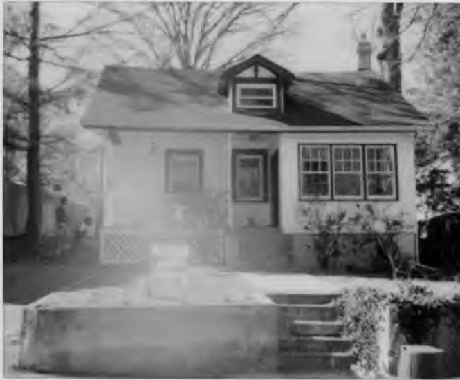
Silver Renovation 7324 Baltimore Ave., Takoma Park ① New brick pier and wood posts 3-17-88
