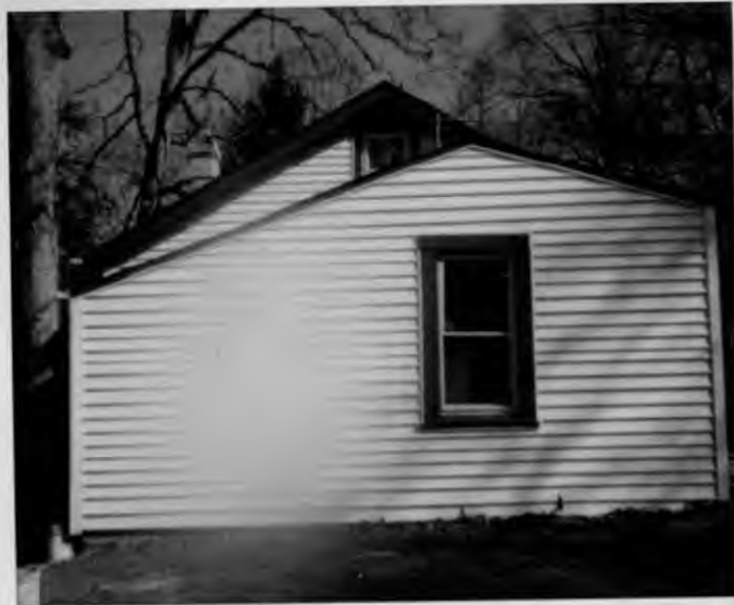
Silver Renovation 7324 Baltimore Ave., Takoma Park ③ New Door & Window to be added 3-17-80
