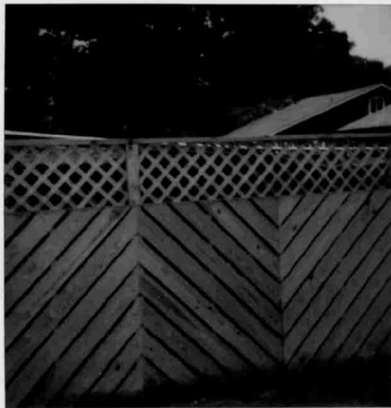
MIDDLE SECTION OF FENCE PLASTIC TARPULIN LOOMING THROUGH LATTICE
