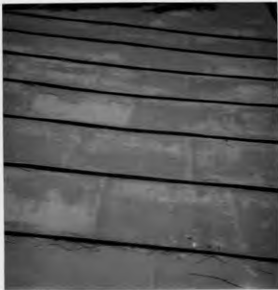
Typical Standing Seam Note: in need of paint
