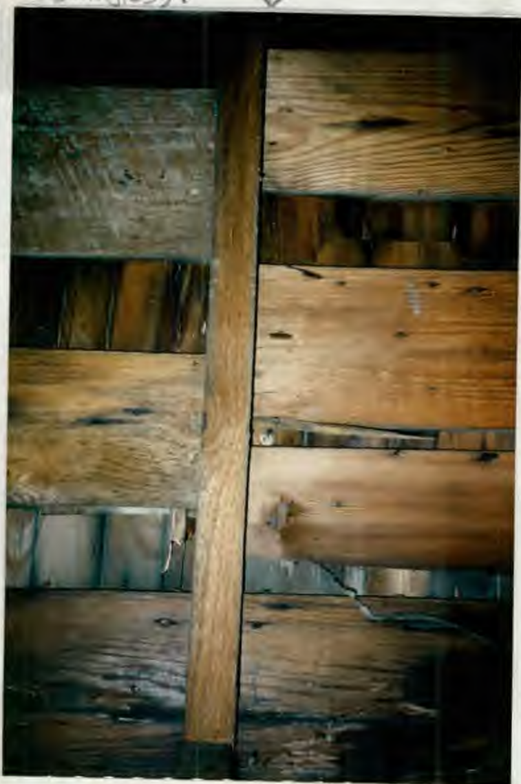
(41) Roof on south side viewed from interior. (Note wood shingles overlapping -- under newer asphalt shingles). ↓
