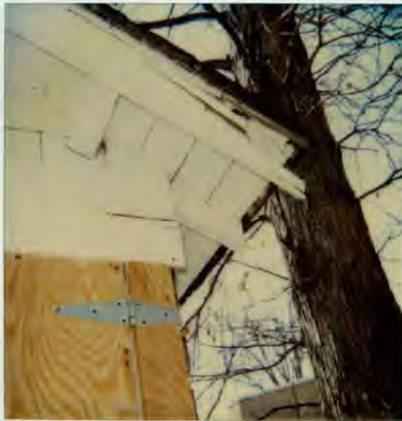
Roof damage of old garage
