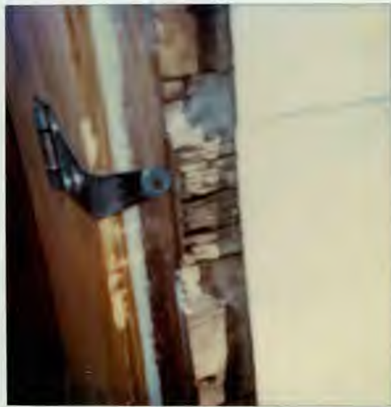
Termite damage on Garage
