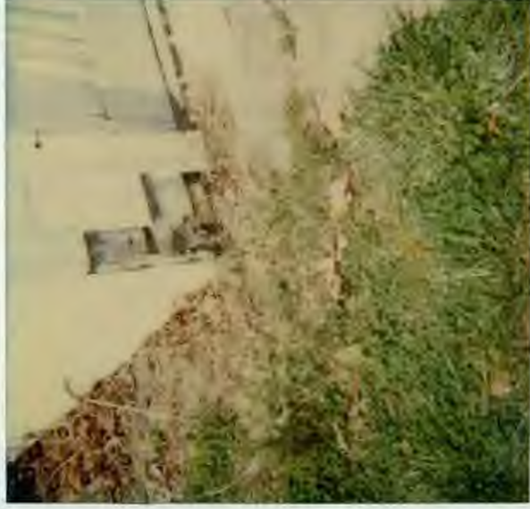
Permite Damage on base
