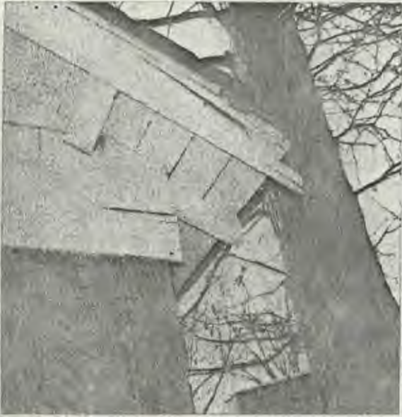
Roof damage on old garage
