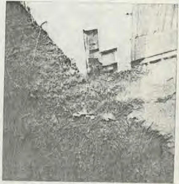
termite damage on garage
