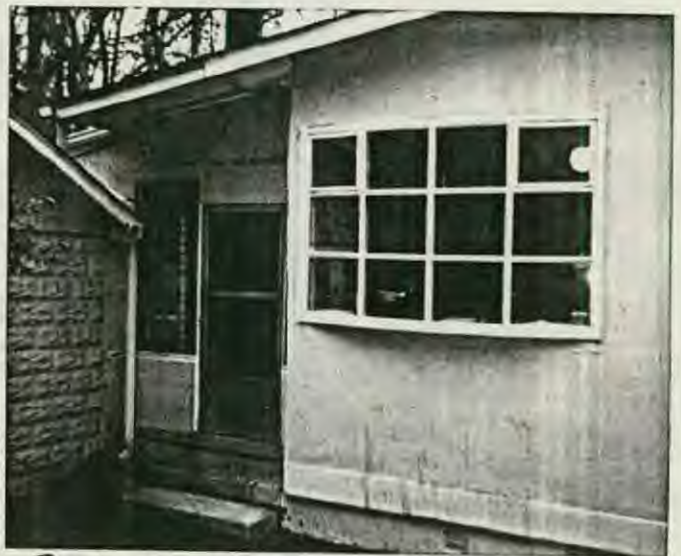
BAY TO BE REPLACED WITH (3) DOUBLE HUNG WINDOWS, PORCH WALL TO BE MODIFIED. SEE 9/1.
