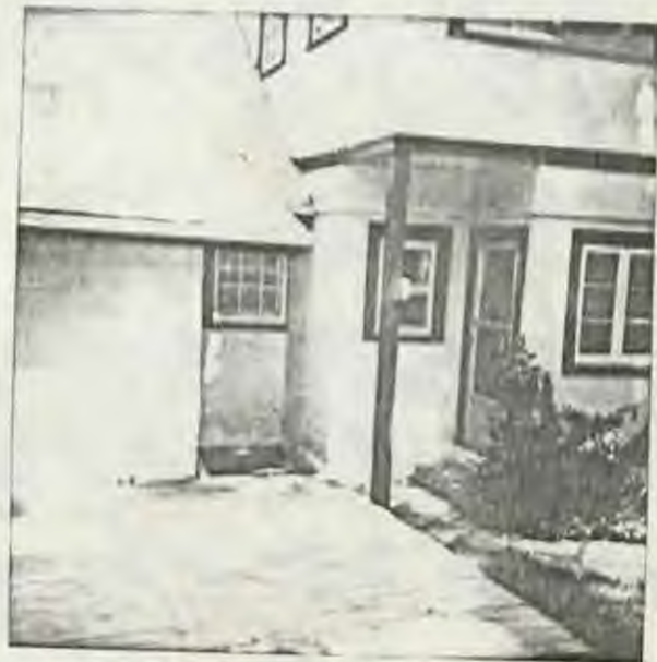
Area to be filled in by addition Rear side of 7321 Willow Ave.
