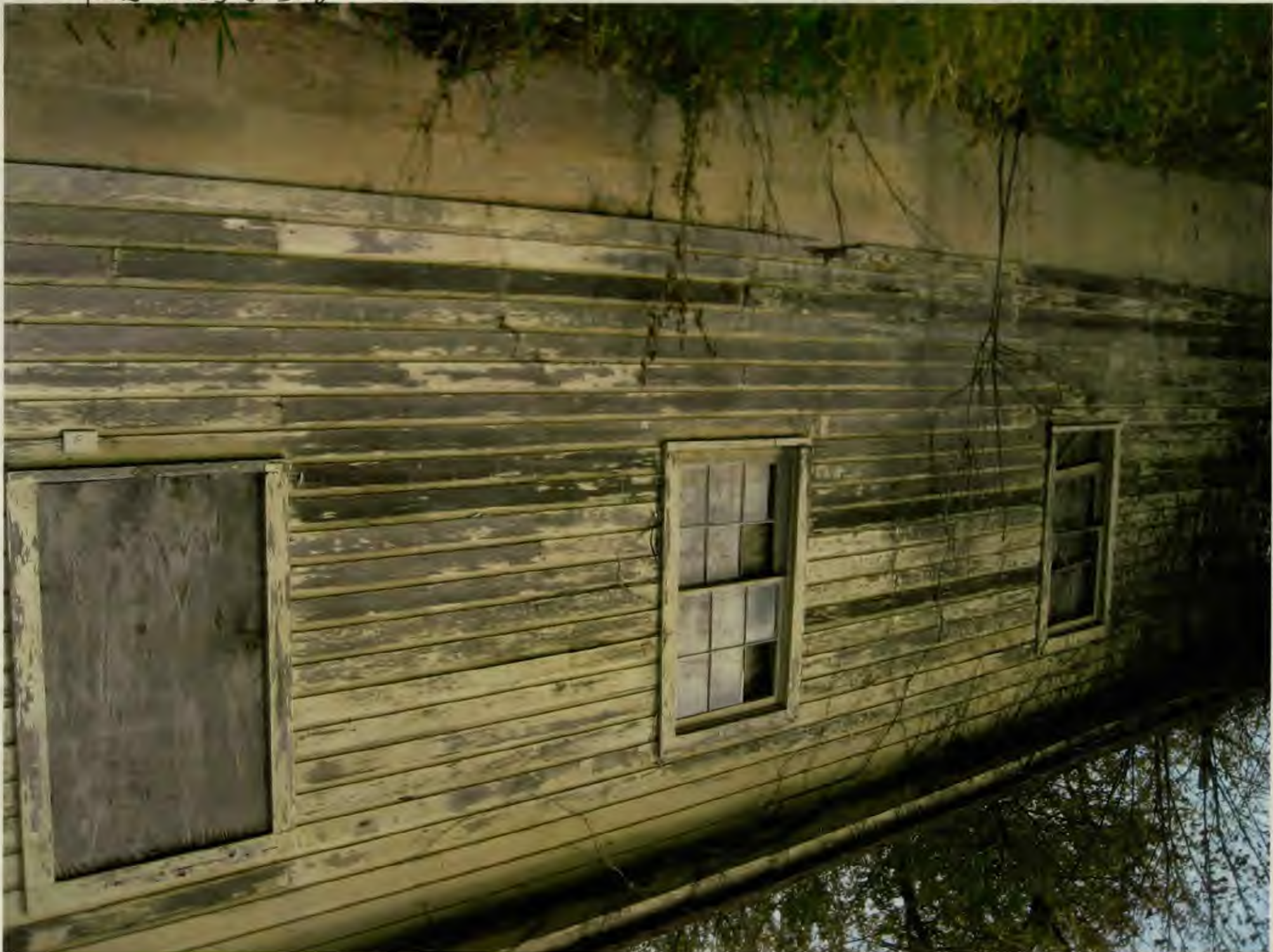
Rear of frame. 5109
