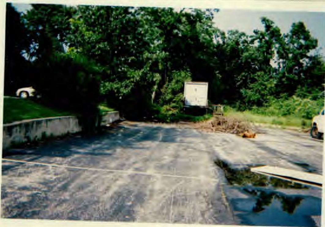
Rear parking area and retaining wall. Trailer storage with small wooden deck.
