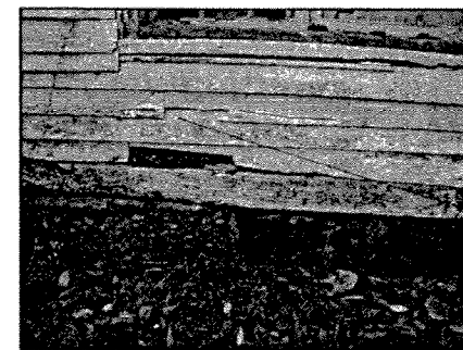
RESTORE AREAS OF SIDING AND TRIM ON THE WEST END TRANSITION BETWEEN CONCRETE AND FIELD STONE FOUNDATION
