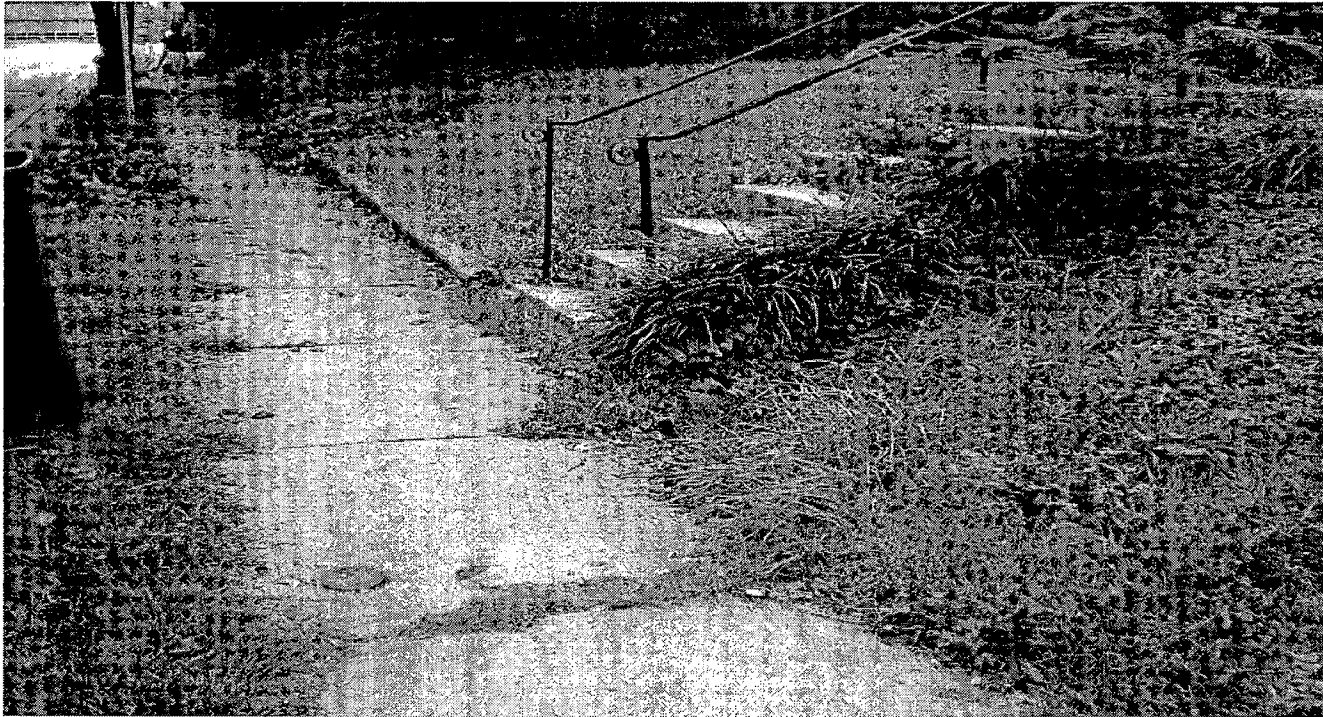
15 Philadelphia Ave. There is a wall to the left of the stairs and none to the right.
