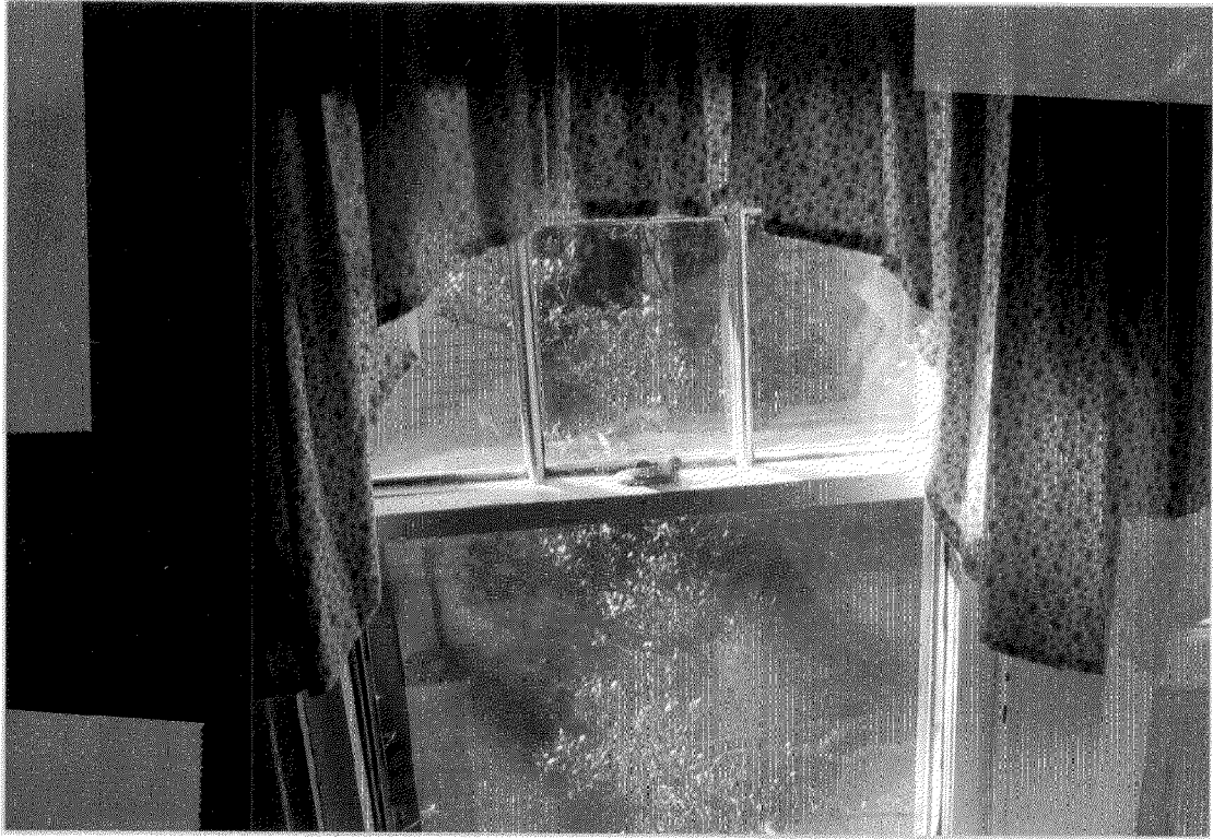
WINDOW ON LEFT SIDE. NOTE TOP OF BOTTOM SASH IS HIGHER ON RIGHT THAN ON LEFT IN CLOSED POSITION.
