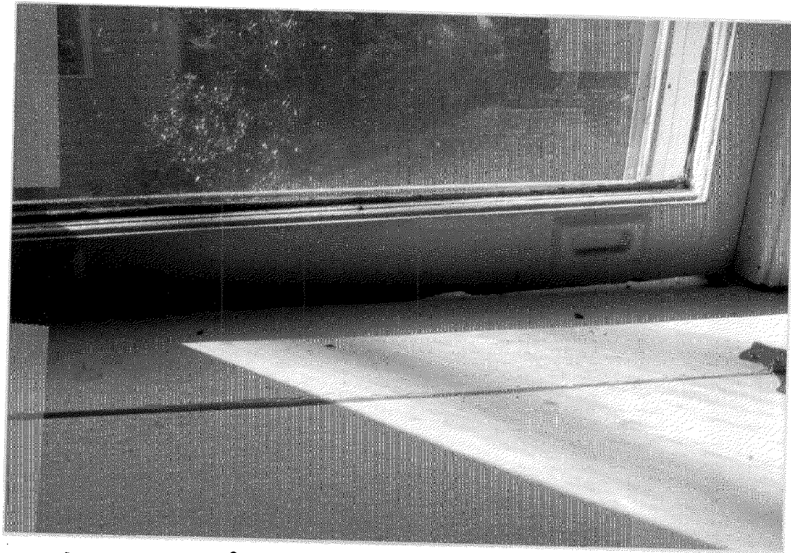
BOTTOM OF SAME WINDOW. NOTE GAP BOTTOM RIGHT.
