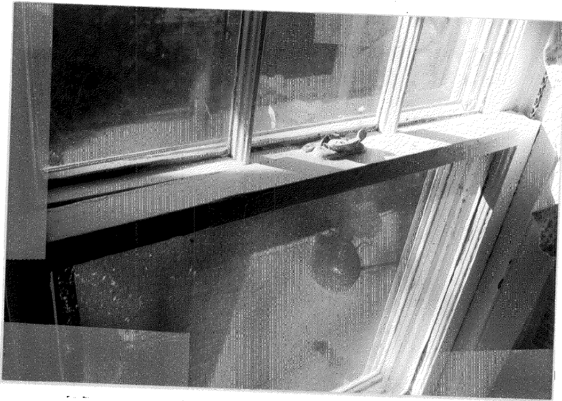
WINDOW ON LEFT SIDE BEING REPLACED AT CUSTOMER'S REQUEST. NOTE WINDOW IS HIGHER ON RIGHT THAN ON LEFT WITH WINDOW CLOSED.
