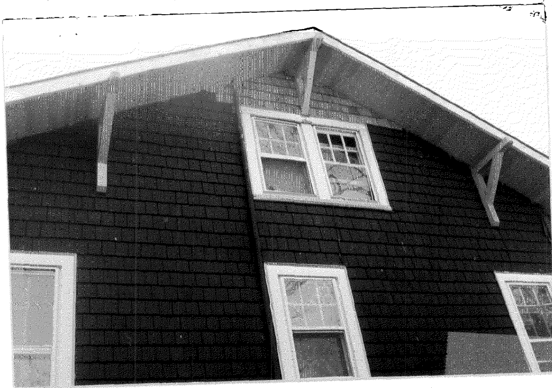
CURRENT WINDOWS 2ND FLR RIGHT ELEVATION. THESE WINDOWS ARE BADLY DAMAGED INSIDE AND CAN'T BE REPAIRED.
