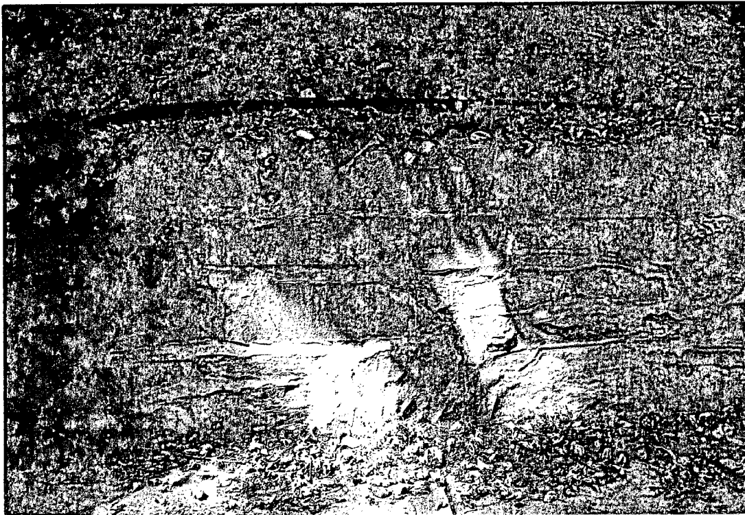
Detail: Front retaining wall, left side (missing base work)
