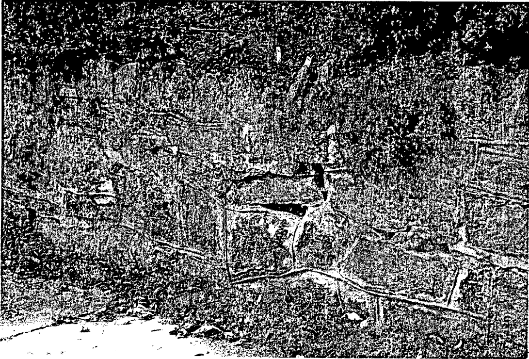
Detail: Front retaining wall, left side (missing stones)
