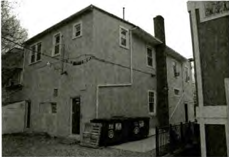
7040 CARROLL AVE EXISTING REAR/LEFT FACADE The Area of Work includes all windows shown
