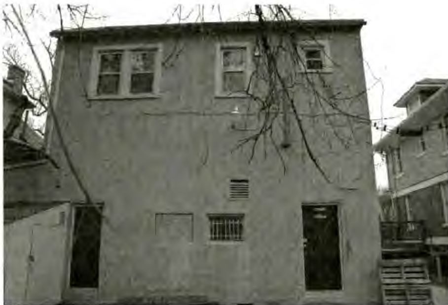
7040 CARROLL AVE EXISTING REAR FACADE The Area of Work includes all windows shown
