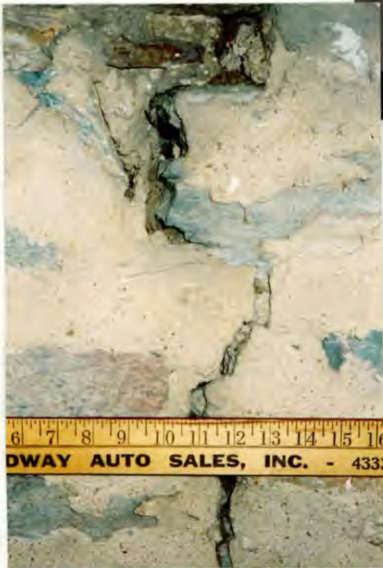
Foundation Crack, Rear Wall
