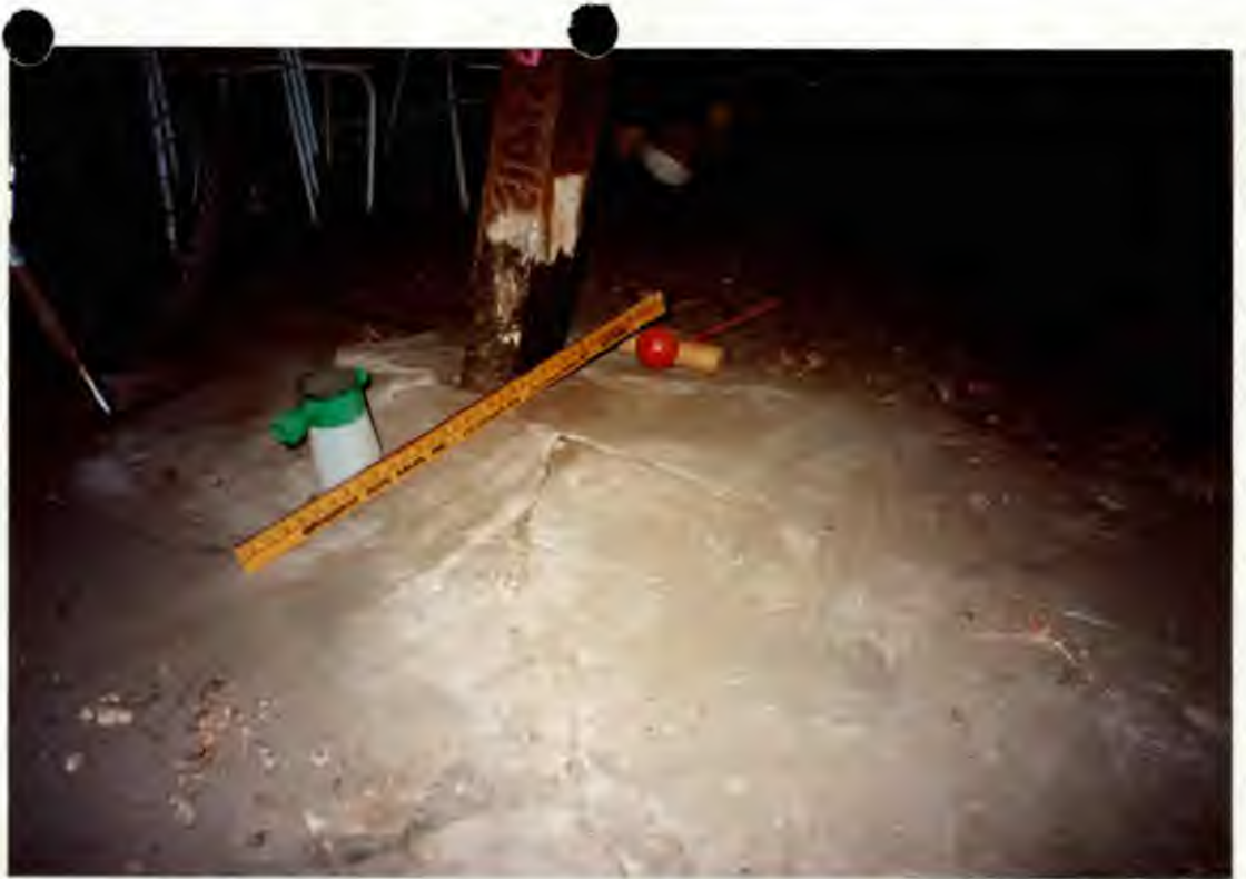
Floor, Cracked and Settled
