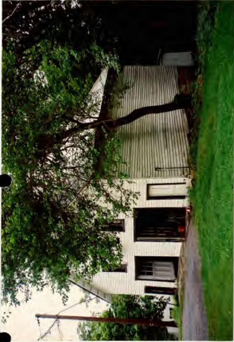
Tree impinging on Garage
