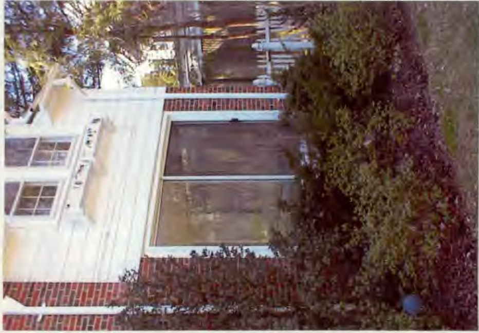
⑩B CLOSE-UP OF FRONT OF SUNROOM. THE EXISTING LANDSCAPING CONCEALS THE BOTTOM OF THE STRUCTURE.
