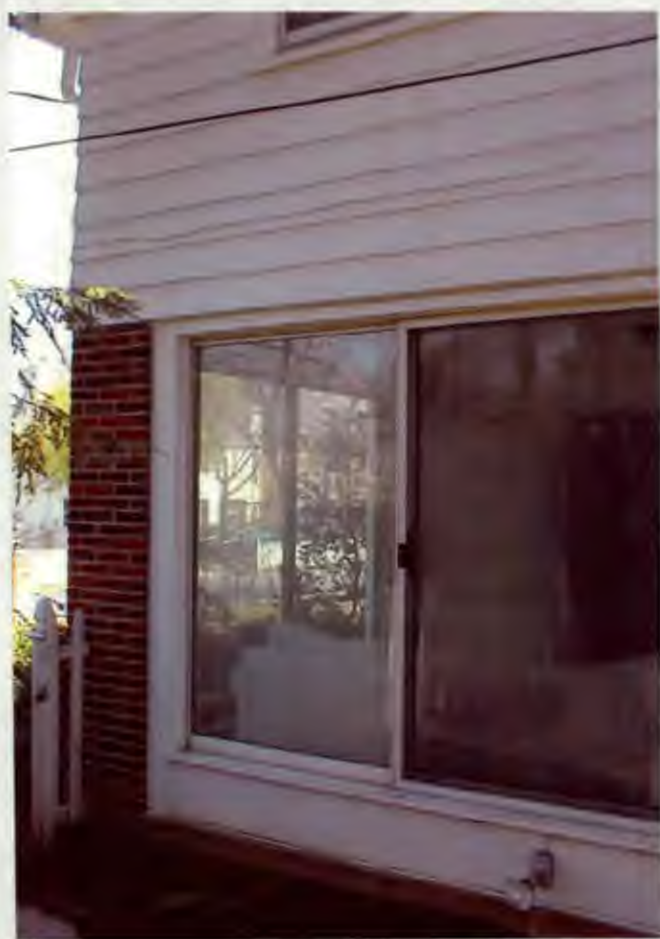
⑧ DETAILED VIEW OF SUNROOM WITH OLD SLIDING GLASS DOORS USED AS WINDOWS.
