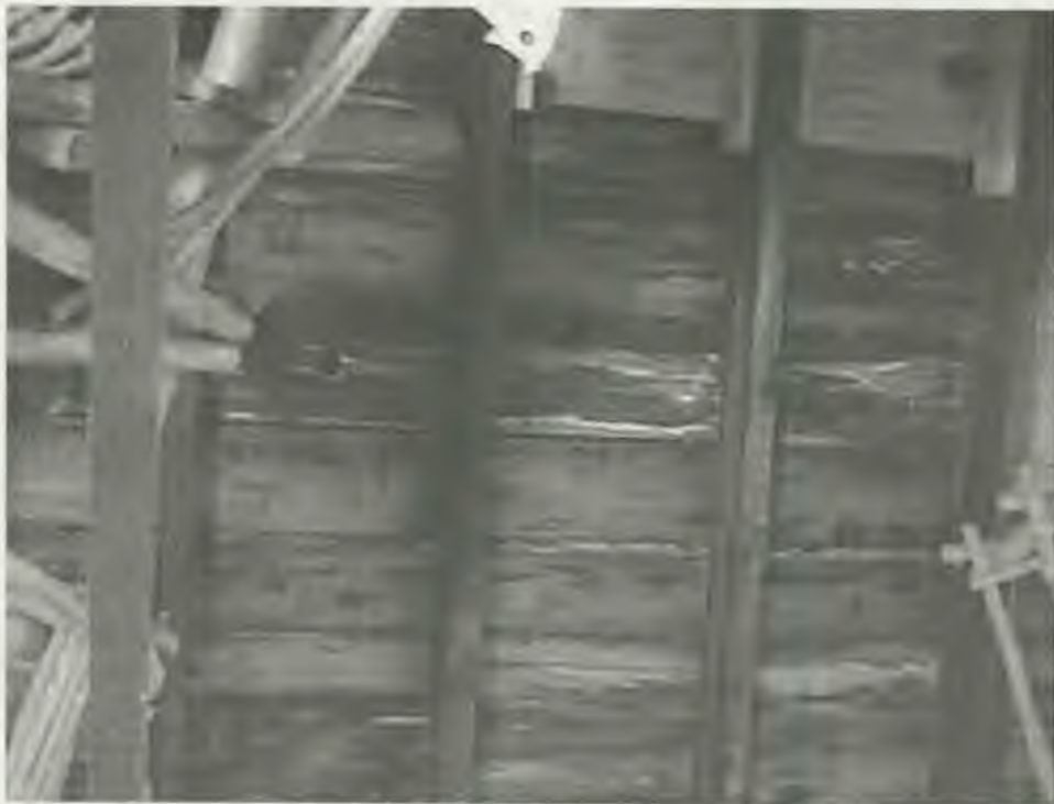
Interior water damage
