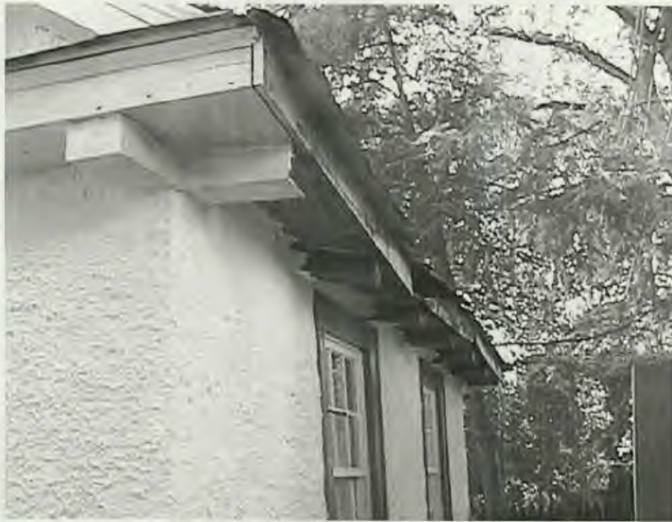
Rear of garage (visible water damage)
