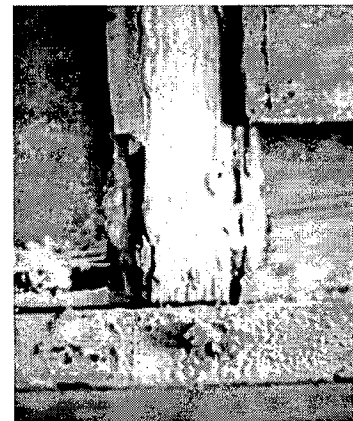
This historic double-hung window has many layers of paint, some cracked and missing putty, slight separation at the joints, broken sash cords, and one cracked pane. Photo: NPS files.
