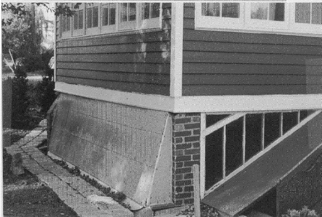
Close view of subgreenhouse - buttress pier (far end), reconstructed front pier, roofing covering of window well
