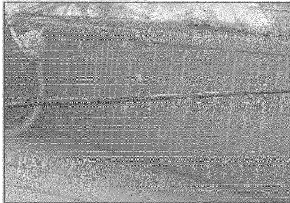
7 Damage at Northwest Eave N/S
